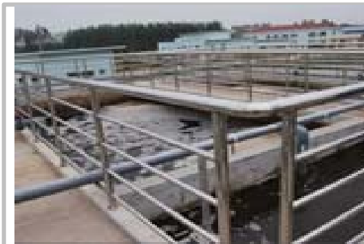
Leachate system process
