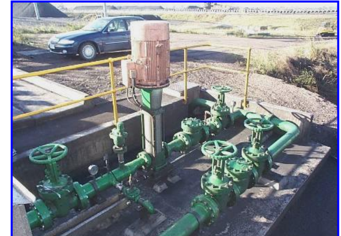
Specification & Scope of Work Preparation Design and Installation of 20 litre/sec high pressure water booster pump and 600m pipeline
