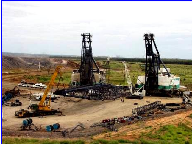
Heavy Lift Specification and Execution 190T Three Crane Lift to transfer a Dragline Boom
